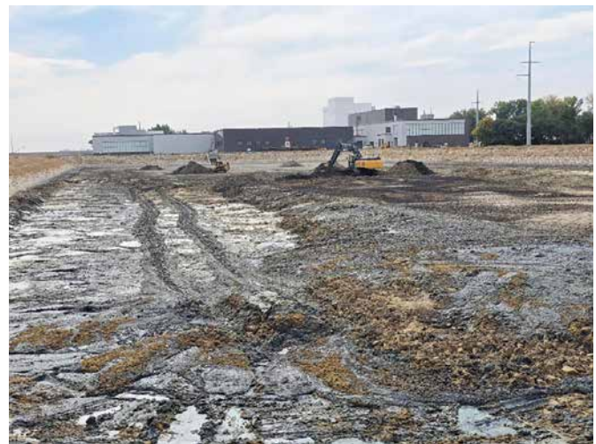
Figure 9: Excavating equipment preparing water treatment sludge (residuals) for removal from a settling pond at the BPWTP.
